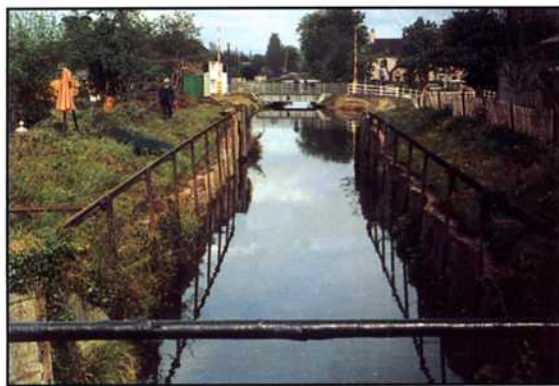
The turf sided lock at Aldermaston before restoration with a scalloped brick chamber and old railway tracks to prevent barges floating out of the main chamber. ©BCC.
