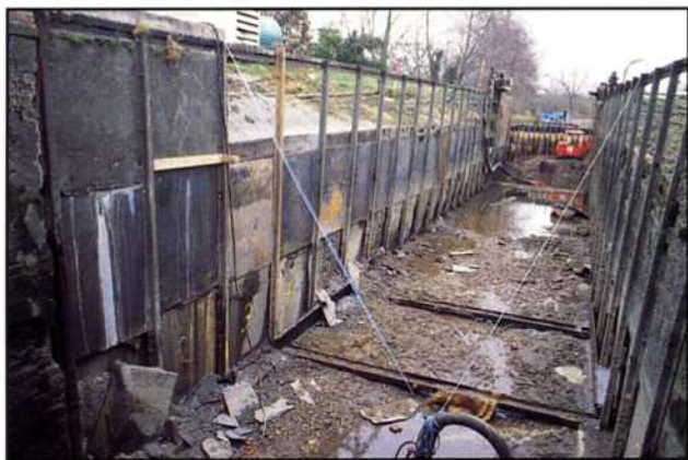
Garston Lock during refurbishment in January 1997. The profile of the sloping turf sides can be seen behind the slate sheathing boards retained by redundant broad gauge tracks from the Great Western Railway. © WA.
