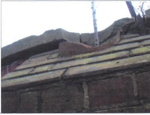
Figure 3 The top of the butters with the rim of the top section of pipe showing
