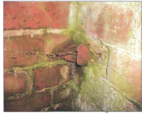
Figure 4 The outlet pipe in close-up. This one is chipped but is thought to be near to its original length
