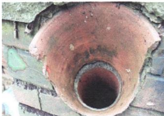
Figure 2 The top of a pipe, rim broken, showing its 'flowerpot' shape and its junction with the glazed down pipe.
