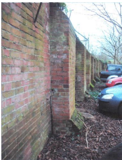
Figure 1 One of the buttresses outside the wall, side outlet two thirds of the way down, hard against the wall. The lower courses are not keyed into the wall.
